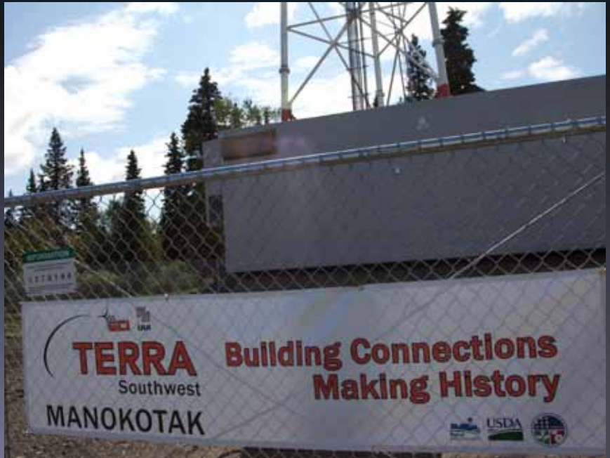
Microwave tower and Shelter in Manokotak, AK
